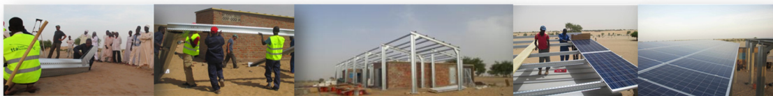
Construction and Commissioning of 3 Solar Photovoltaic microgrids in Chad on a Turn-key Basis, including techno-economic-social feasibility
